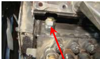
Return Line From the P-7100 Pump Figure 53
