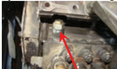
Figure 56 Return Line From the P-7100 Pump
